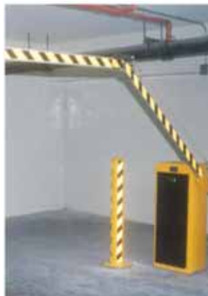
Car Park Gate control
